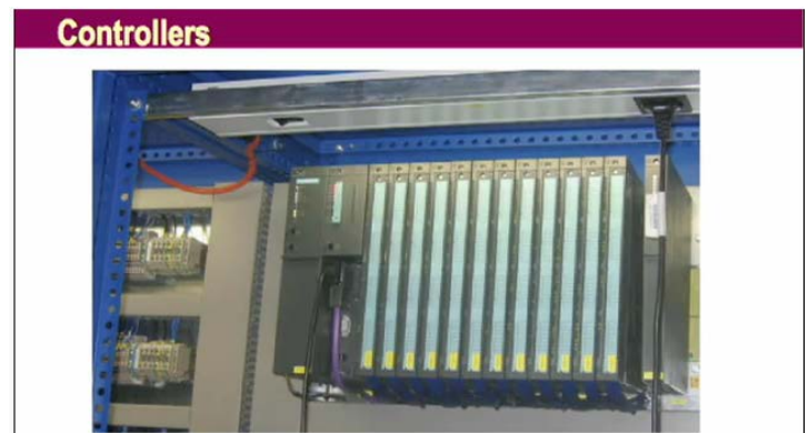
Figure 9: PLC Controllers exploited by Stuxnet
